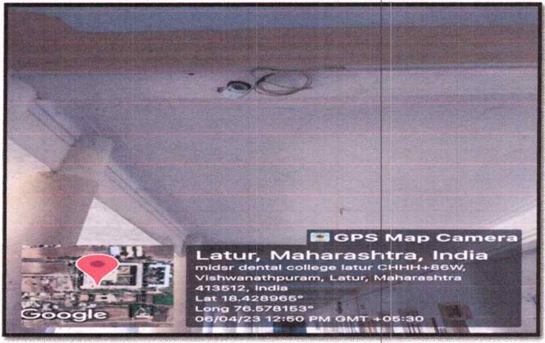
CCTV Surveillance inside the campus
