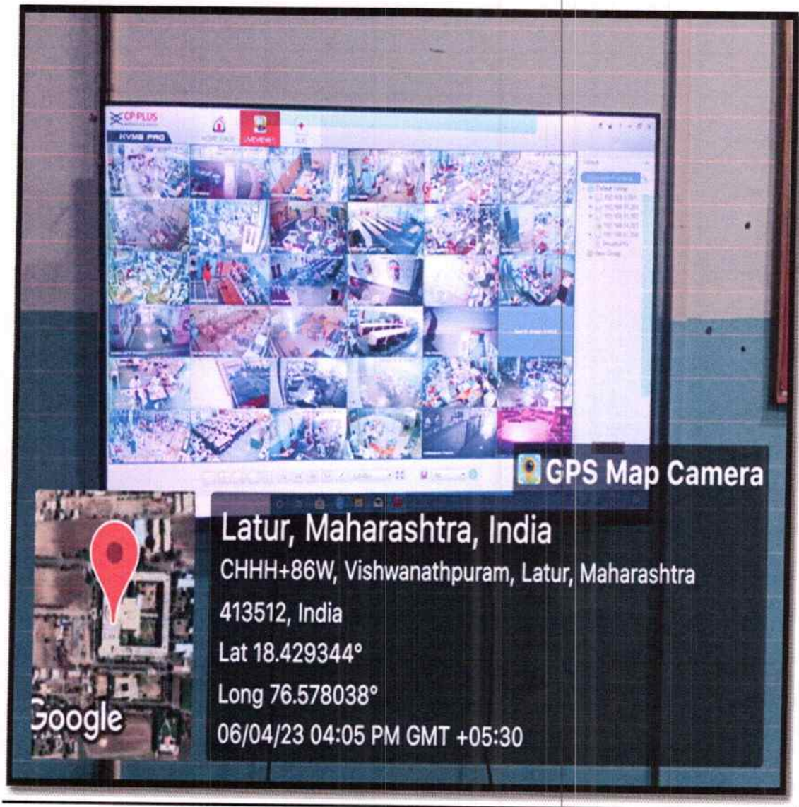
CCTV camera's surveillance in Principal's office
