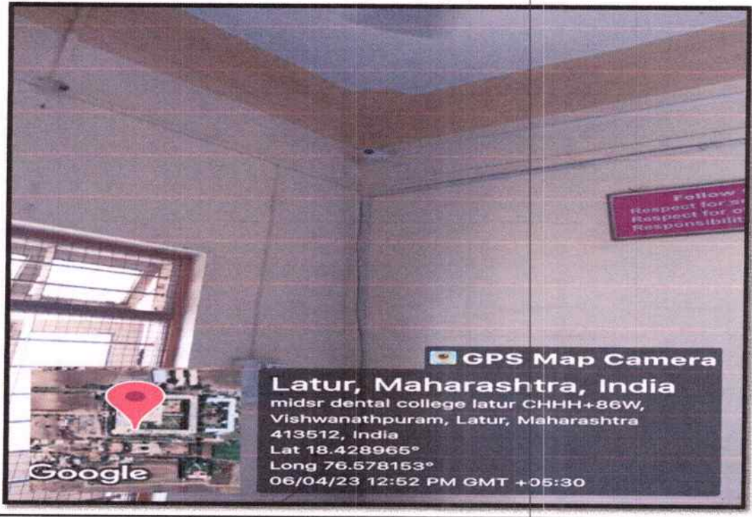
CCTV Surveillance inside the campus
