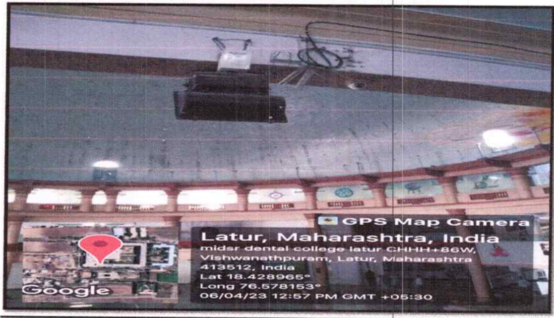
CCTV Surveillance inside the campus
