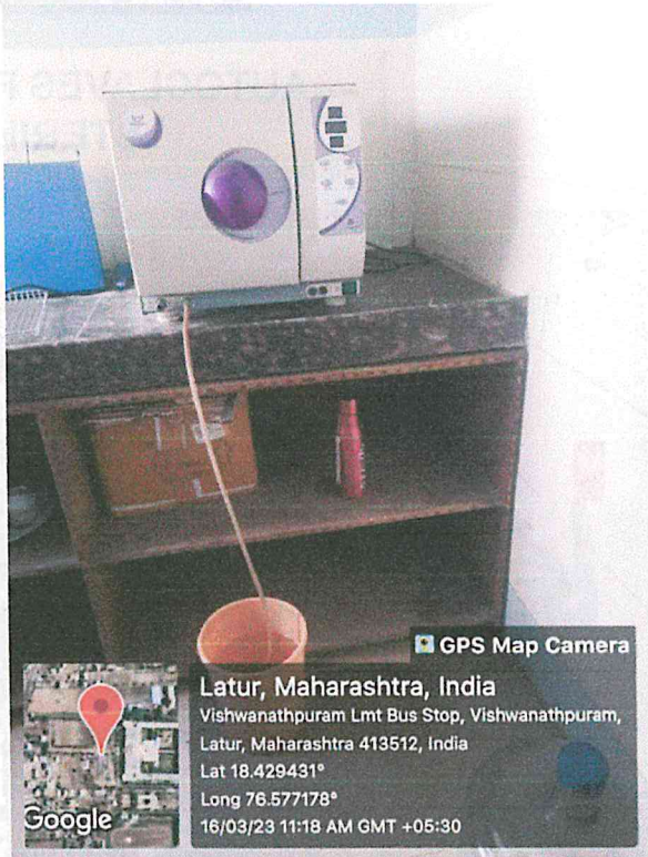
AUTOCLAVES FOR BULK INSTRUMENT STERILIZATION VACUUM (FRONT LOADING)
